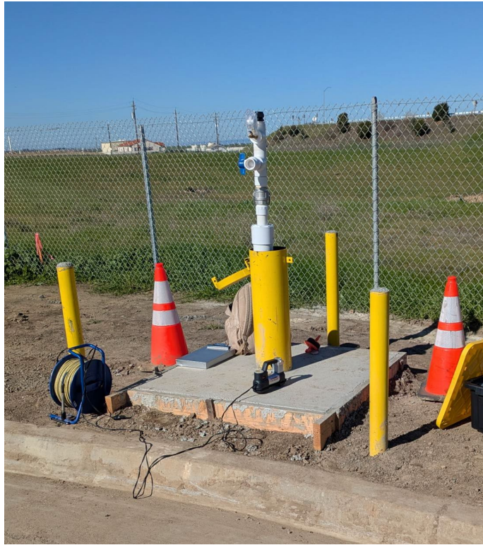
Figure 4. Wellhead Manifold and Datalogging Pressure Transducer
