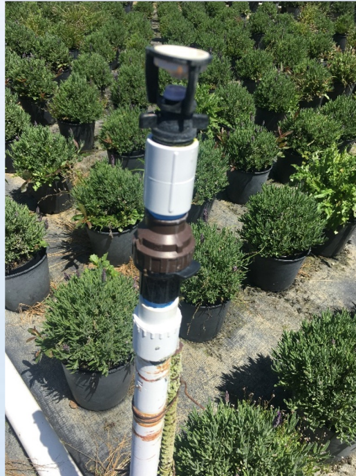
Sprinkler check valves
